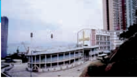
Foundation works of the development site at Ka Wai Man Road is in progress. 位於加惠民道之地盤地基工程現正進行。
